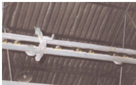
Can cable - transfer
